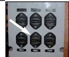
WINDLASS CIRCUIT BREAKER
