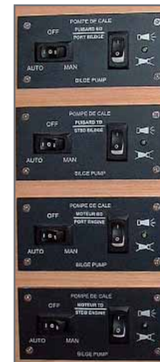
BILGE PUMP PANELS
