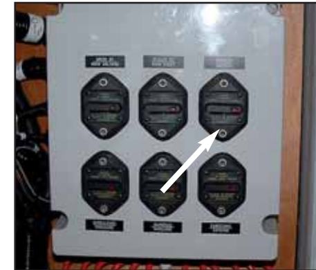
CAPSTANS CIRCUIT BREAKER
