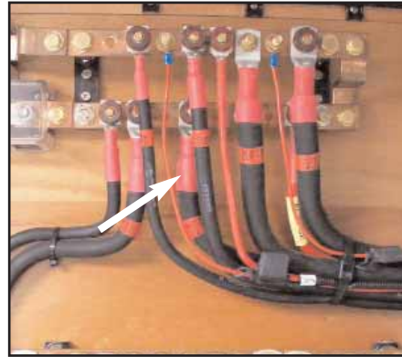
FUSE OF THE SYSTEM (DAVITS)
