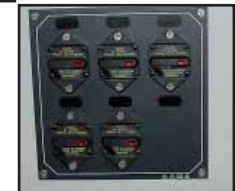
WINDLASS CIRCUIT BREAKER
