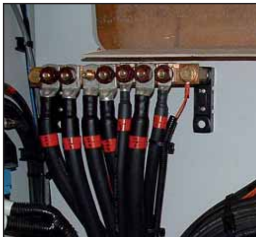
BATTERY BUS BAR
