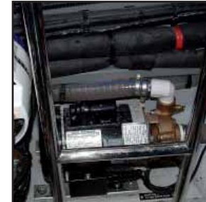
AIR CONDITIONING PUMP
