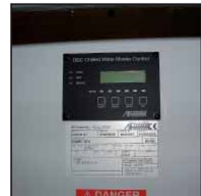
CENTRAL CONTROL PANEL
