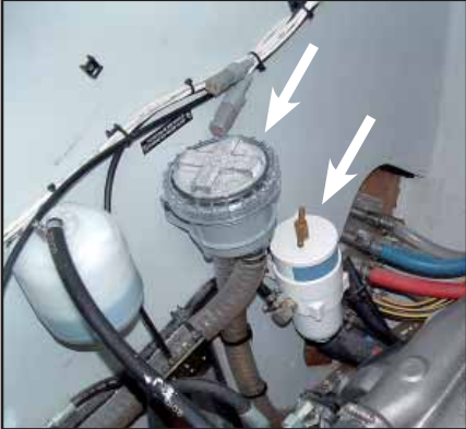
WATER FILTER + FUEL FILTER
