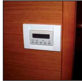
AIR CONDITIONING CONTROL
